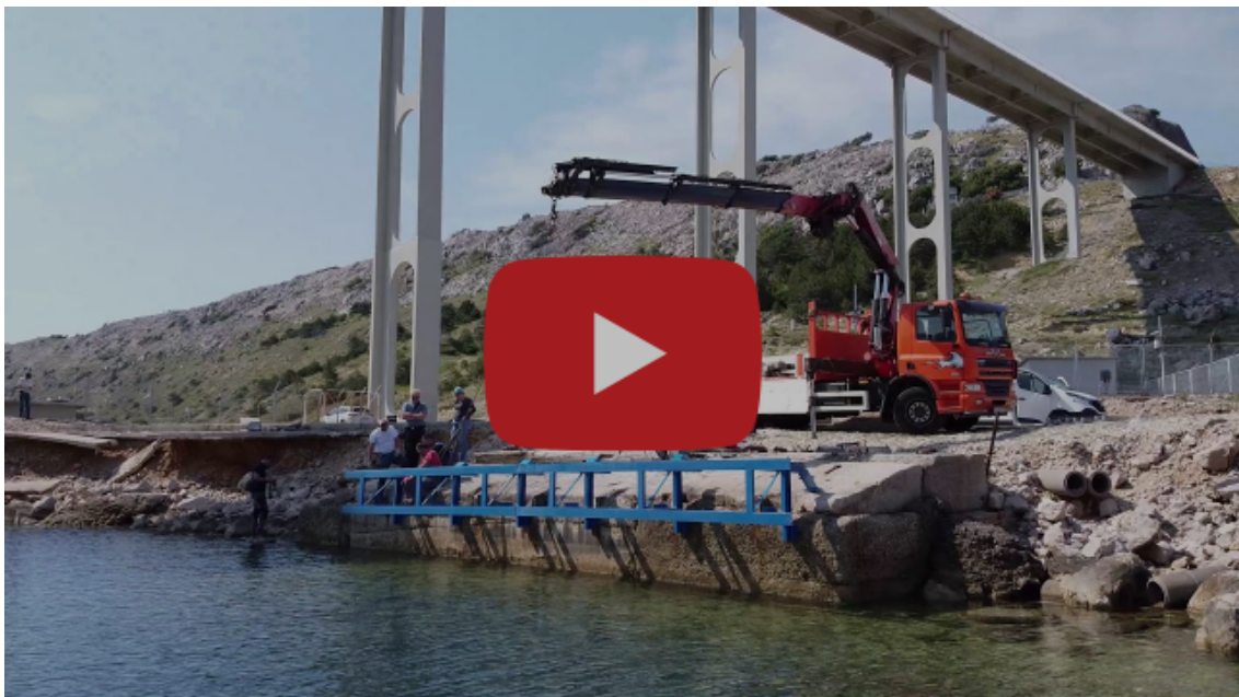
Deployment of EnDurCrete elements at the Krk Bridge demonstration site in Croatia.
